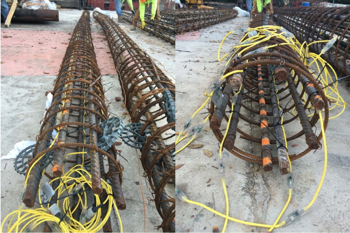
Figure 2.6 Top end of piles C1 (left) and L1 (right) reinforcement cages instrumented with thermal wires.
