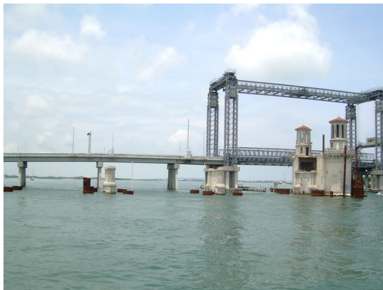
Figure 4.61 West Bascule (Pier 15; right), Piers 14 and 13 moving to the left with four 8-ft shaft casings shown from south looking north during rehabilitation.
