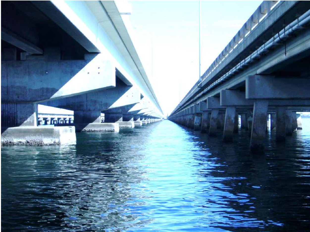
Figure 4.1 Newer cap and column pier design (left); older pile bent piers (right).
