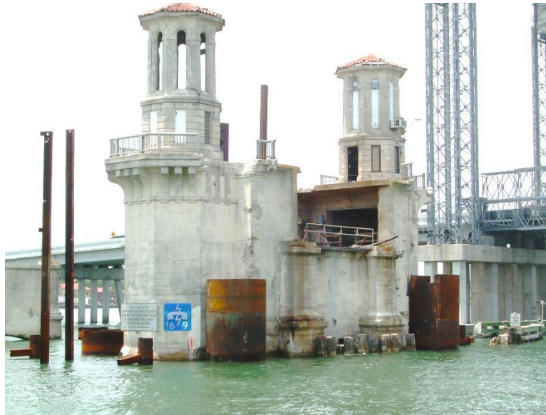
Figure 4.60 West Bascule (Pier 15 implied via plans / Pier 11 via inspection report) during rehabilitation; image taken from SE side looking NW.
