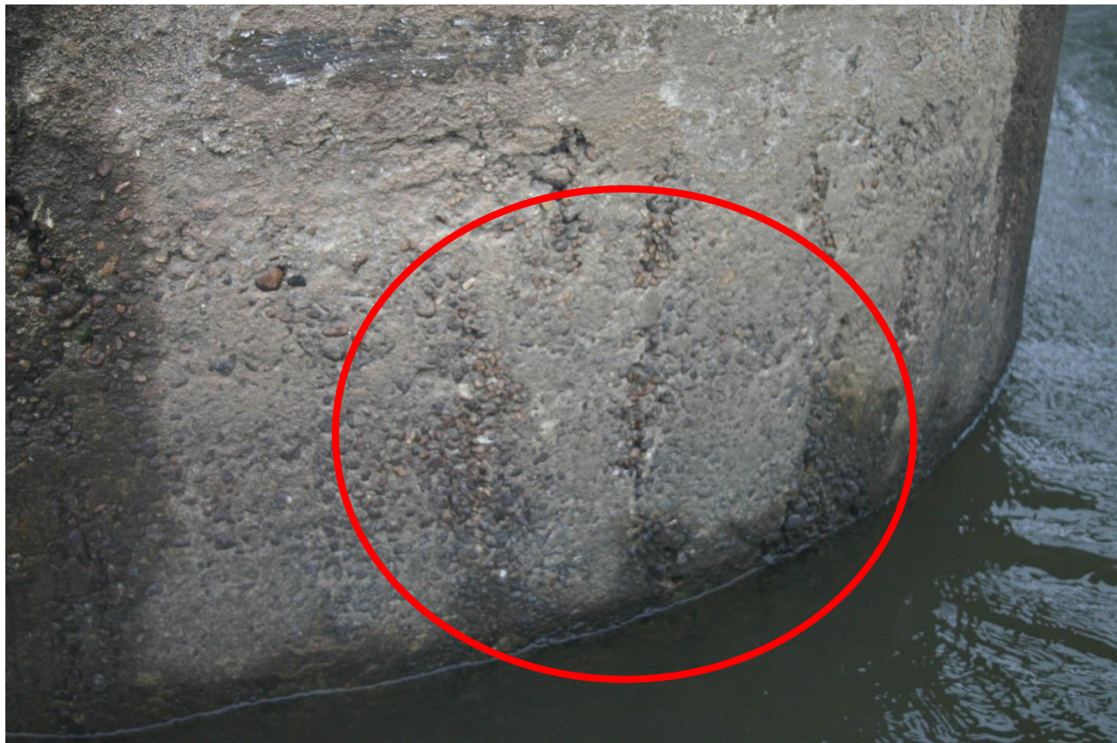
Figure 4.57 West side of test shaft 8, light creases from vertical reinforcement
