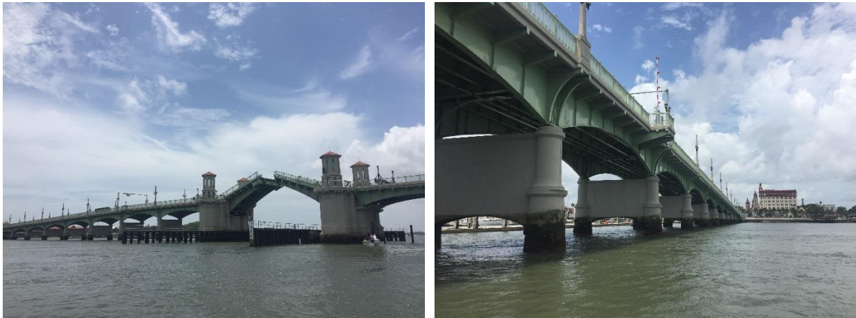
Figure 4.62. Existing main span bascule piers of Bridge of Lions (left); approach spans Pier 14 closest decreasing in number into the distance (per plan numbering).
