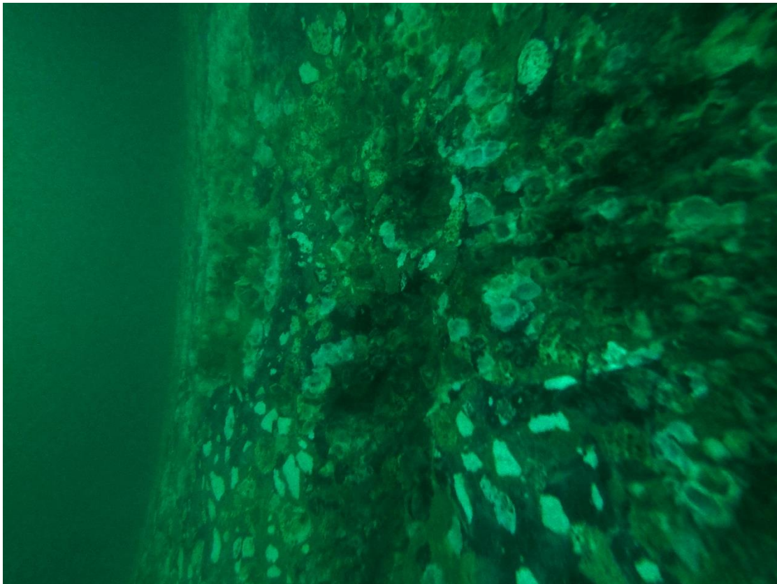
Figure 4.41 Large void found on the south side of 71-4
