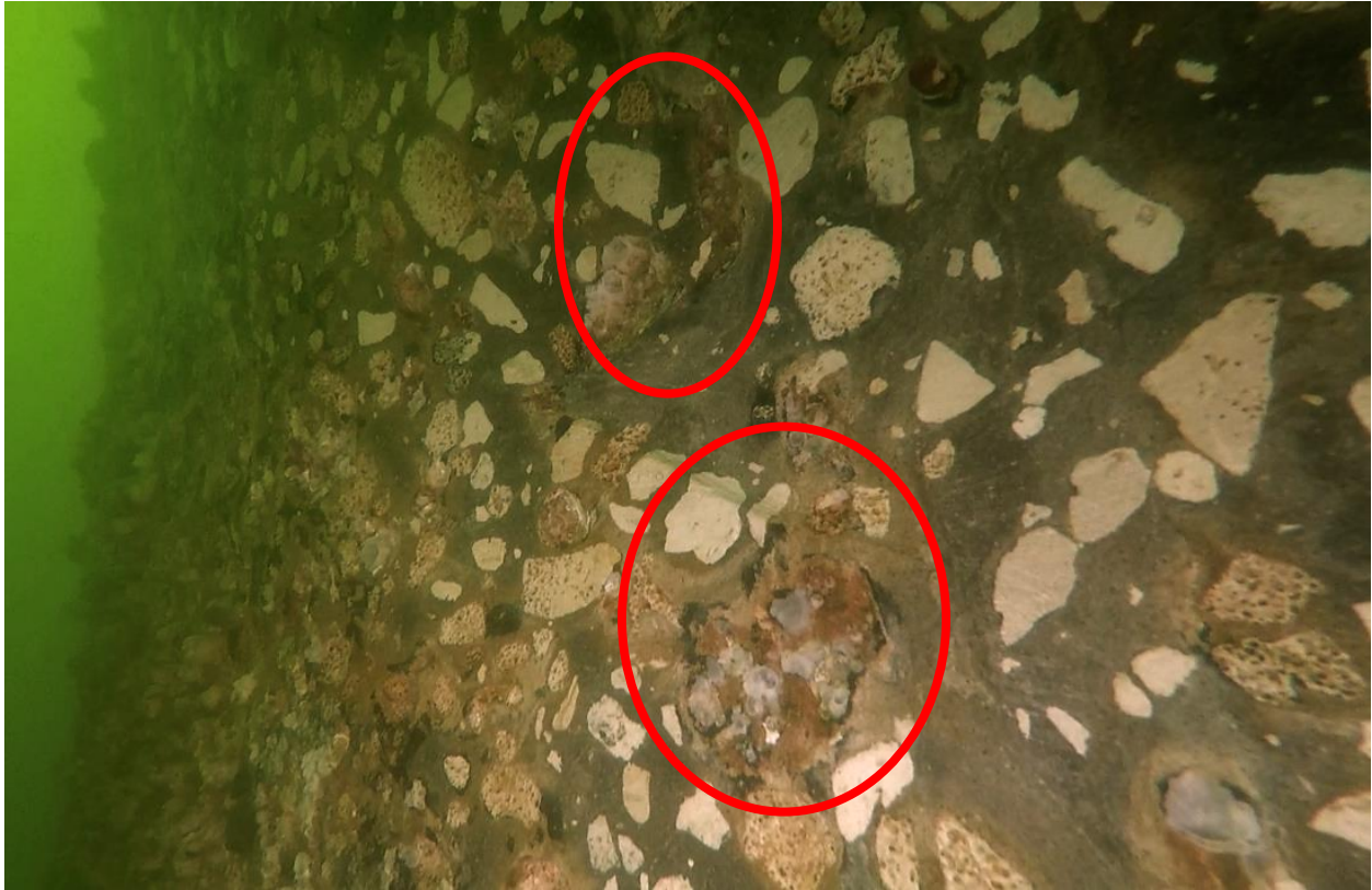
Figure 4.35 Cleaned portion of 84-4 on the southeast side of the shaft, circled sections indicate small voids in concrete filled by barnacles
